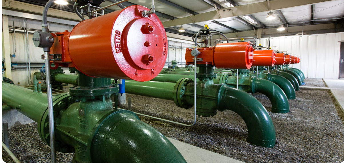
Northwest Pipeline located in Sumas, Washington.
