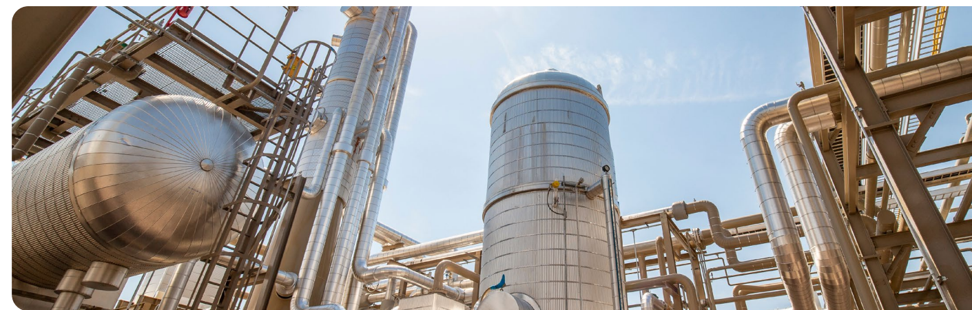
Fort Lupton Cryogenic Facility near Fort Lupton, Colorado.
