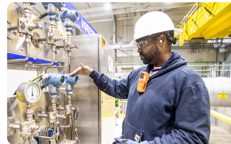
Josh Moore, Operations Technician at Transco Station 185 in Manassas, Virginia.
