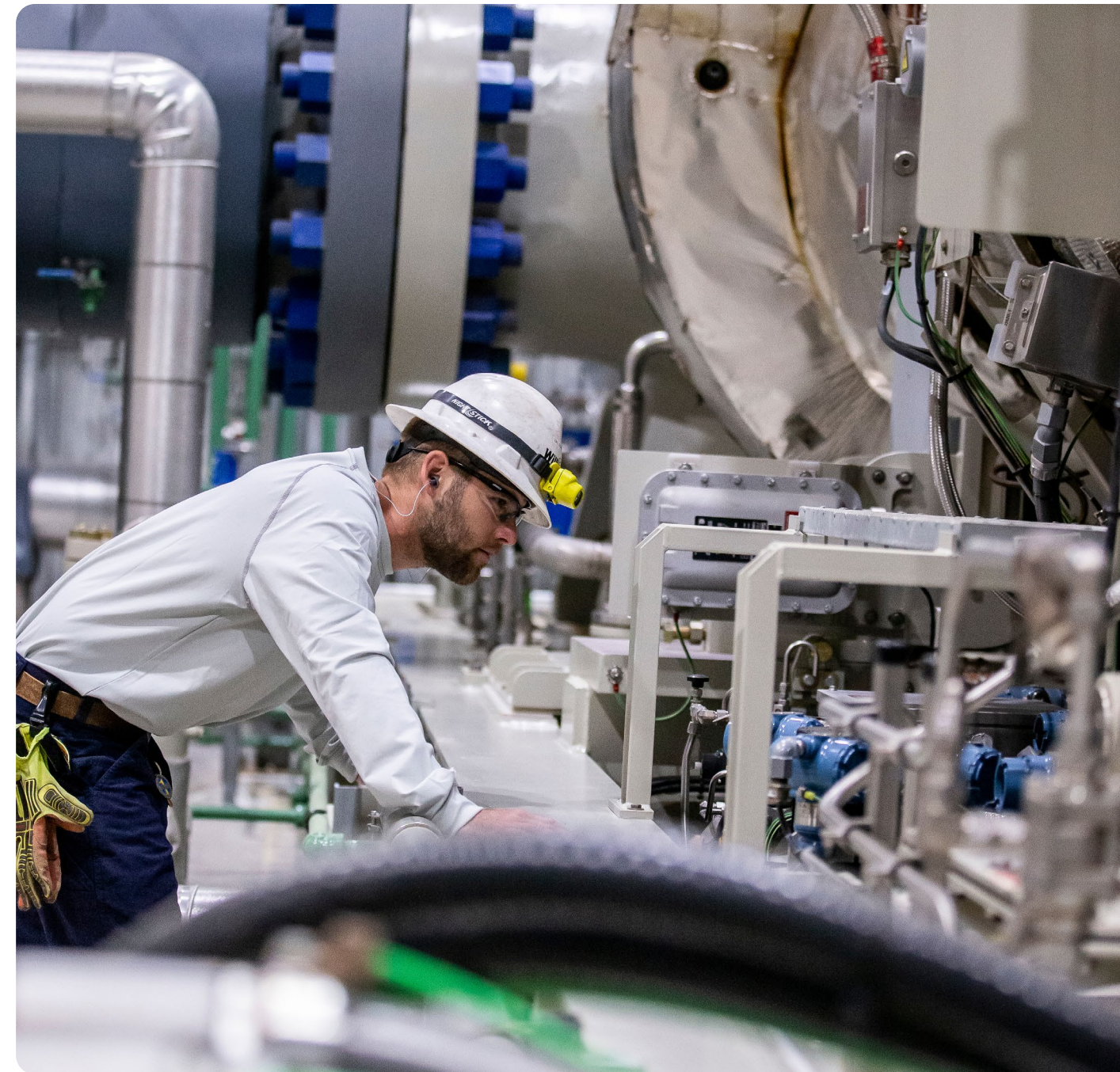
Zac Compton, Operations Technician, at the Transco Pipeline Station 165 in Virginia.
