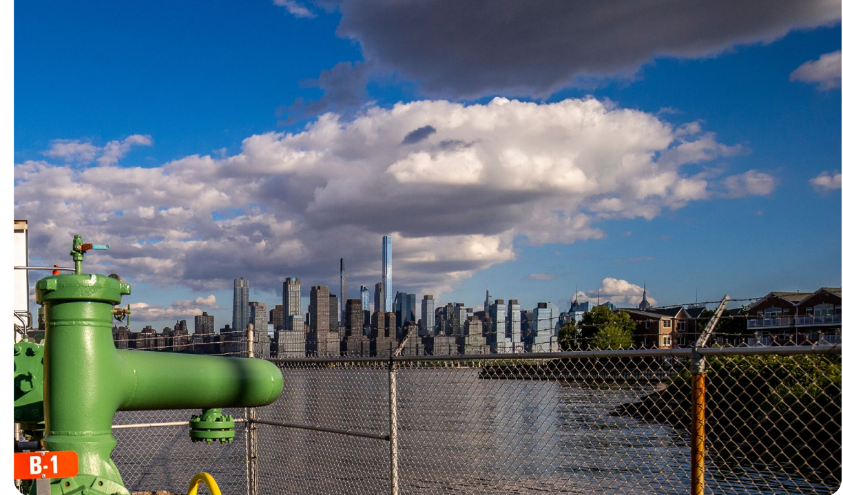
72nd Street Valve Site in North Bergen, New Jersey.
