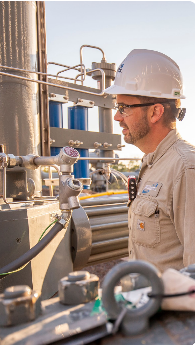
Doug Schloegel, Maintenance Coordinator at the Transco Pipeline Station 610 in Millersville, Pennsylvania.
