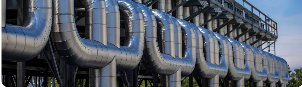
Transco Station 175 in Scottsville, Virginia.
