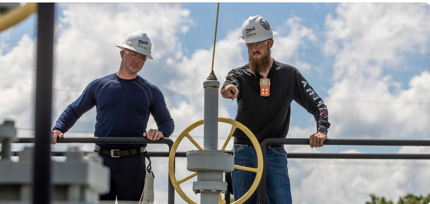
Jeff King, Senior Operations Manager, and Michael Watkins, Training Specialist at the Transco Pipeline Station 145 in North Carolina.
