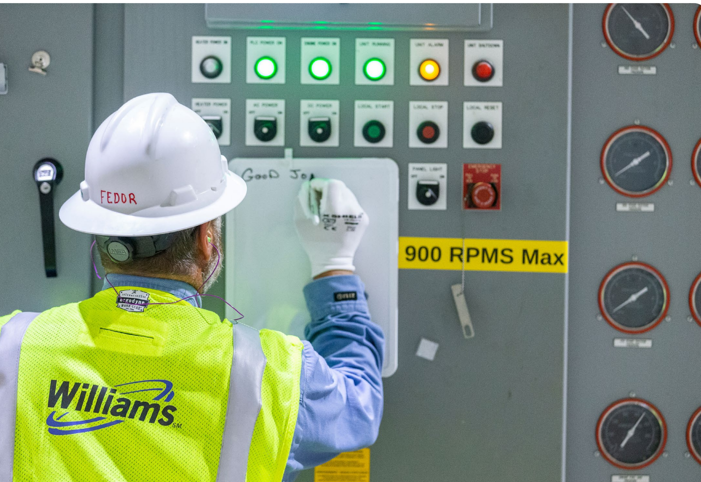
Chris Fedor, Operations Technician at the MacNew Compressor Station in Hop Bottom, Pennsylvania.
