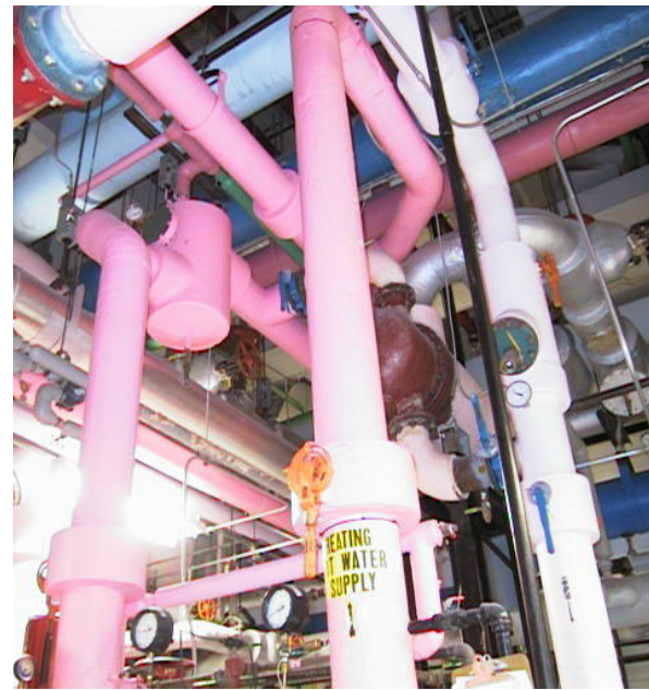
Exceptionally Maintained Mechanical Rooms
