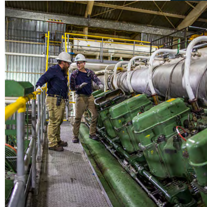
Operations Technicians Joshua L. and Gunnar N. at the Mount Vernon Compressor Station near Mount Vernon, Washington.
