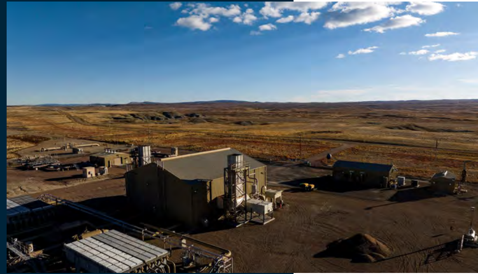
Roberson Creek Compressor Station in Kemmerer, Wyoming.
