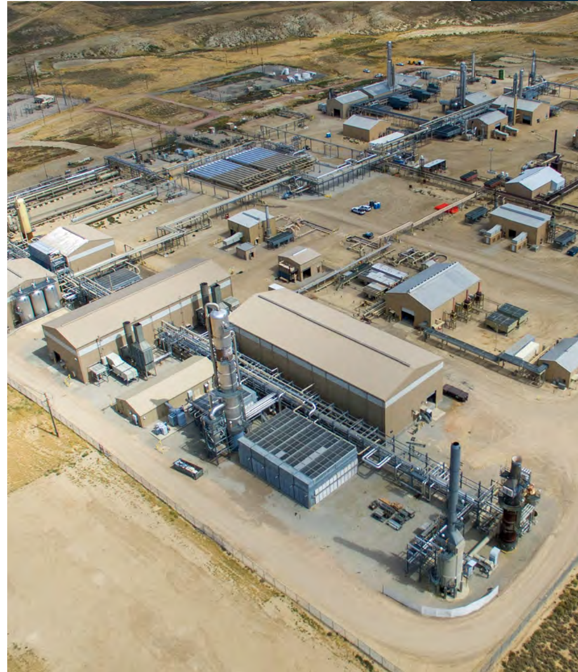
Echo Springs gas plant in Wamsutter, Wyoming.
